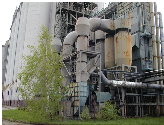
Figure 2. Grain dryer situated next to grain storage complex. Note damaged pipes insulation
