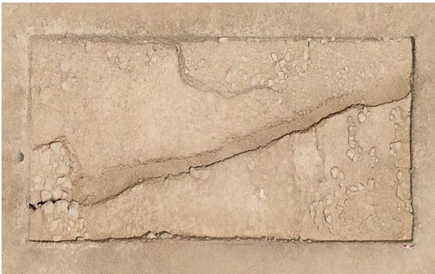
Fig. 11. Architectural structures with a mudbrick residential surface and a continuous subsidence crack in the central section of the site, in view of the Tomb of Darius I (Photo: Younes Zare').
